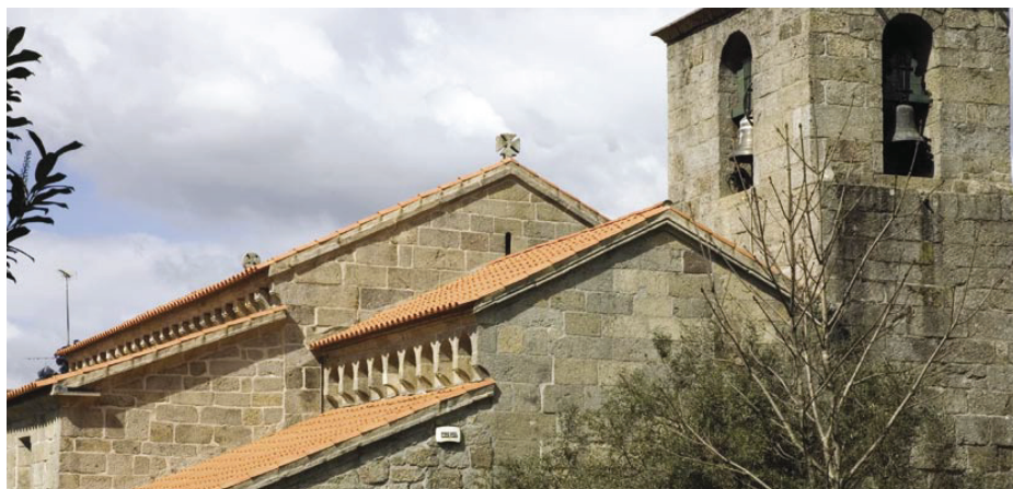
5. The transept presents a cornice over small arches, a solution common to Saint Vincent of Sousa (Felgueiras), Saint Peter of Ferreira (Paços de Ferreira) and a few portions of the Monastery of the Savior of Paço de Sousa (Penafiel).
