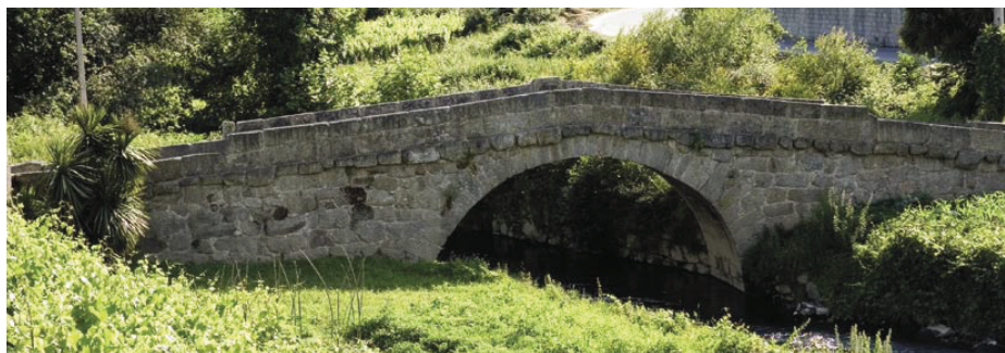
2. Espindo bridge, made of a single arch supported by pillars stemming directly from the banks.
