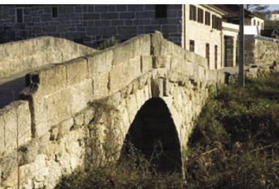
4. At Espindo bridge, the span has forced the elevation of the arch and the positioning of the tray in trestle.
