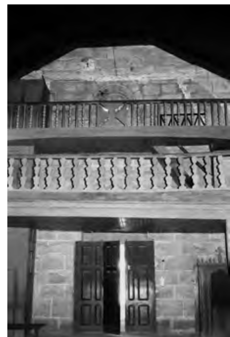
Nave. High choirs before the intervention carried out by the DGEMN (1973). Source: IHRU archive.
