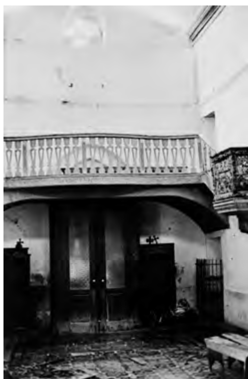
Nave. High choir before the intervention carried out by the DGEMN. Source: IHRU archive.
