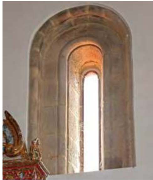
Church. South façade. Nave. Crevice. Interior view.
