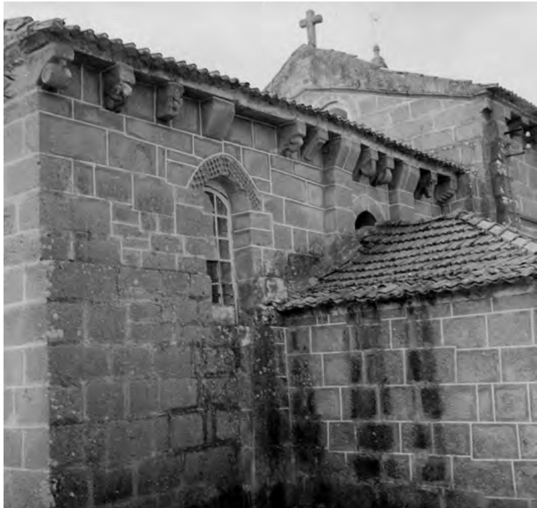
North façade. Chancel after the intervention carried out by the DGEMN (1977). Source: IHRU archive.
