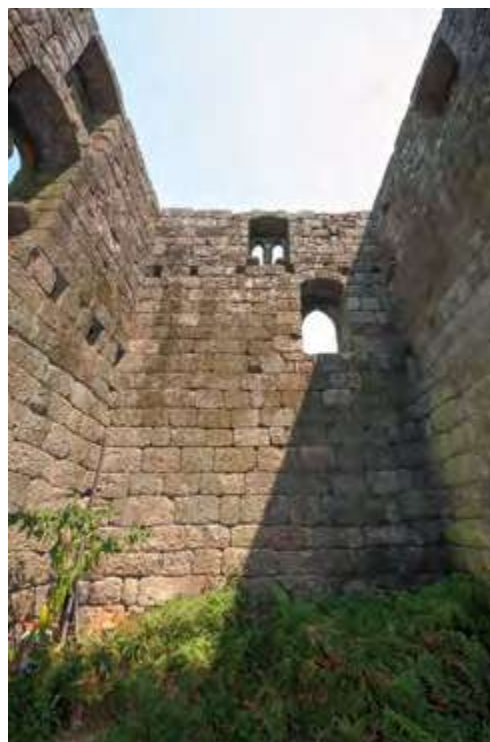
General view of the interior walls before the intervention carried out by the Route of the Romanesque (2014).
