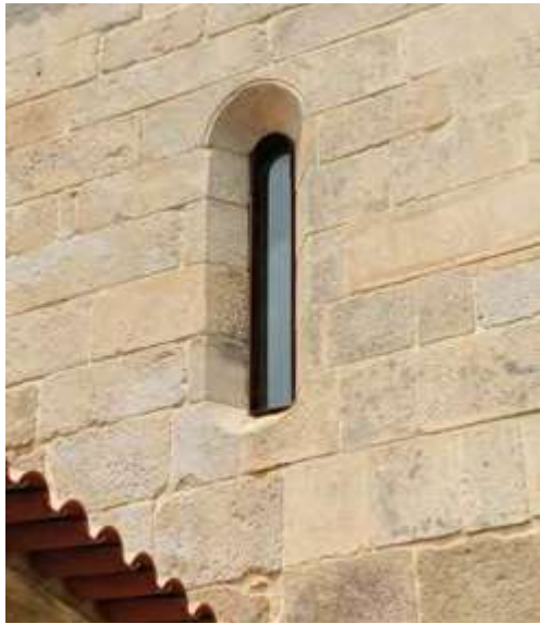
Church. South façade. Nave. Crevice. External view.
