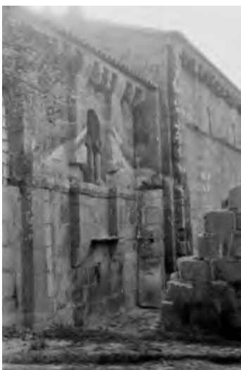
North façade. Chancel before the intervention carried out by the DGEMN (1960). Source: IHRU archive.
