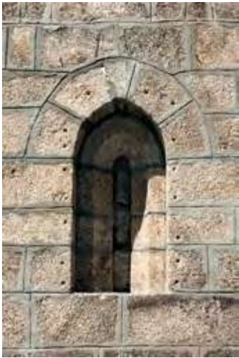
East façade. Crevice.
