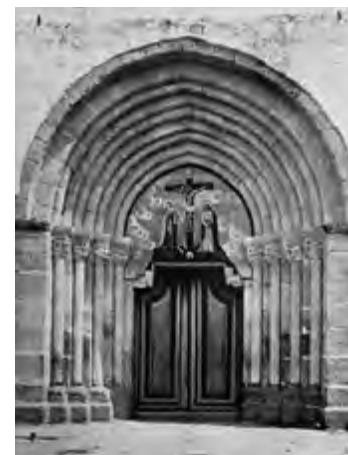
Church. West façade. Portal before the intervention carried out by the DGEMN. Source: DGEMN's Bulletin no. 15.
